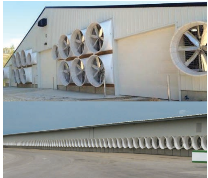
Tunnel and cross ventilated barns can effectively cool cows as long as ECV is met.
