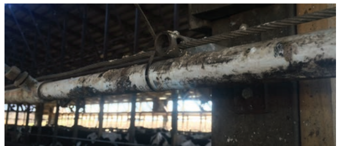
Cable mounted PVC can twist and maintenance is required for nozzle angle adjustment
