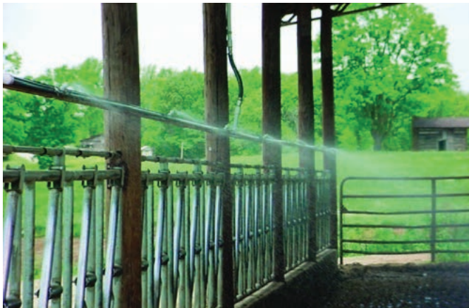
Flex hose connection for water supply line
