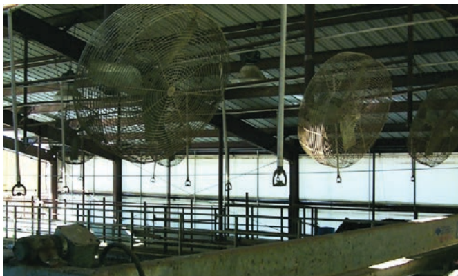
Grid soaker system in holding pens
