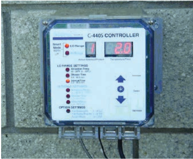
Controller box with 4 solenoid outlets
